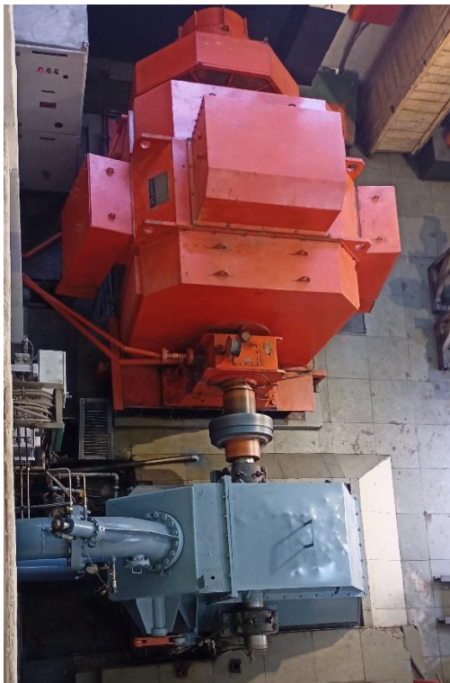
Figure-2: 3 MW Hydro Turbine and Generator inside Power House
