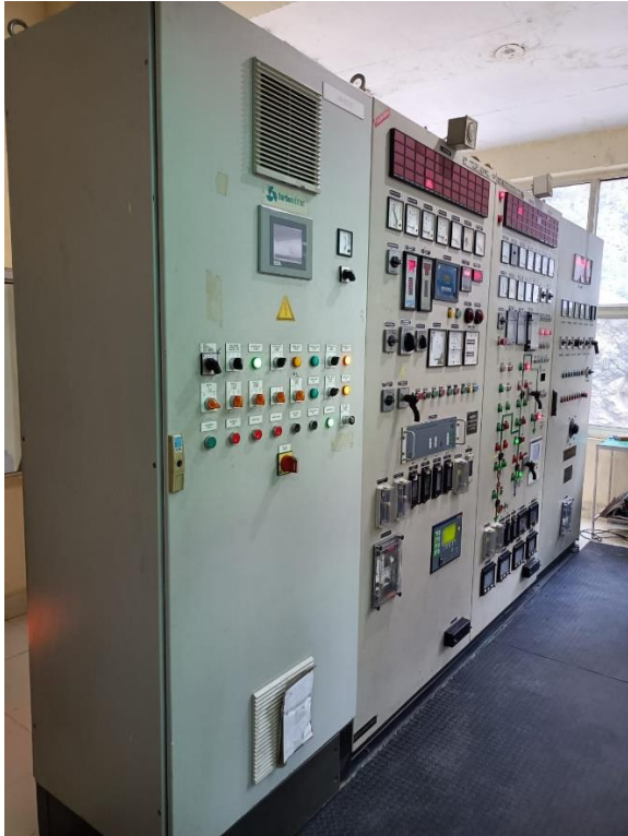
Figure-1: Electric Panel of the Power Plant
